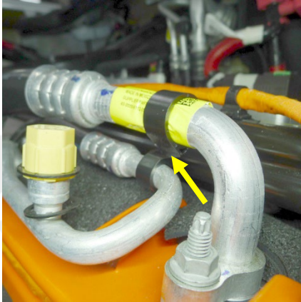
Figure 1 – Support bracket on pipes without foam sleeve
