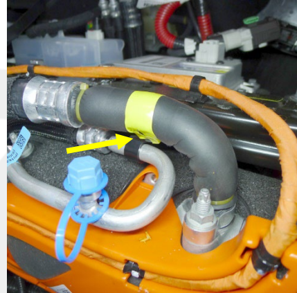
Figure 2 – Support bracket (under tape) on pipes with foam sleeve
