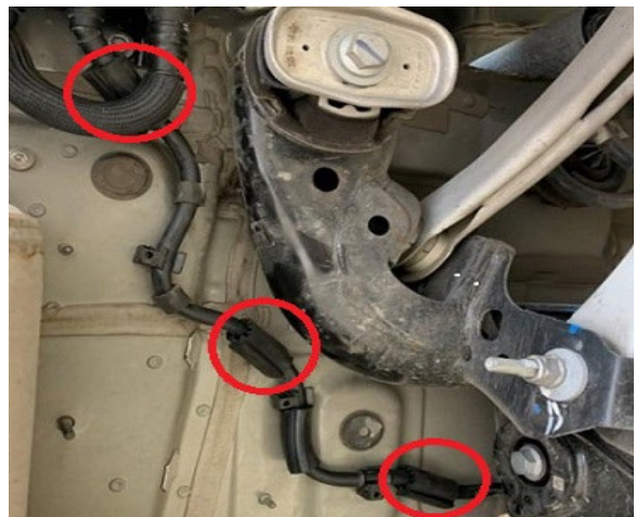
Figure 2: Sleeves installed on the activated charcoal filter line.
