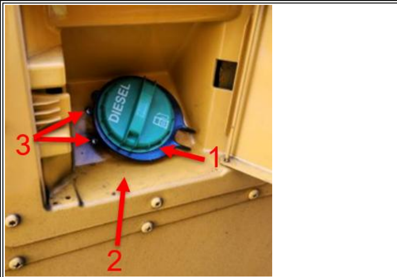
Figure # 1: Fuel Cap Leaking
