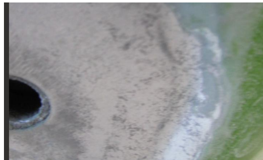
Pitting Found After Sanding Example (Fig. 1)
