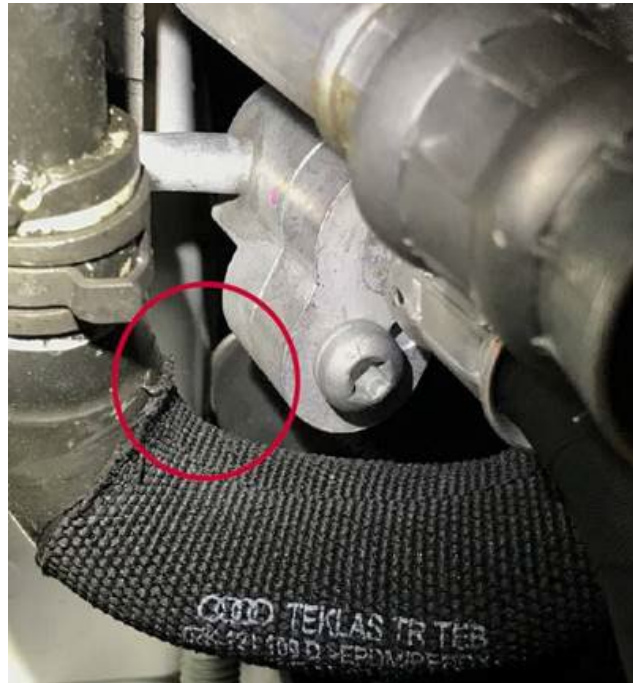
Figure 2. Refrigerant line in contact with longitudinal member.
