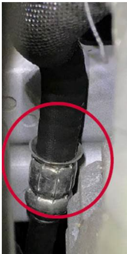
Figure 3. Alternative view of refrigerant line contact with longitudinal member.
