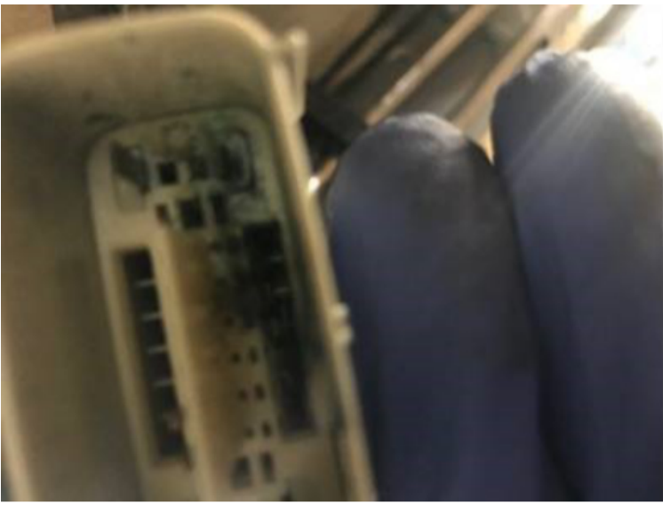
Example of damaged connector at plugged cavity, which may displace the cavity plug, allowing water to enter.
