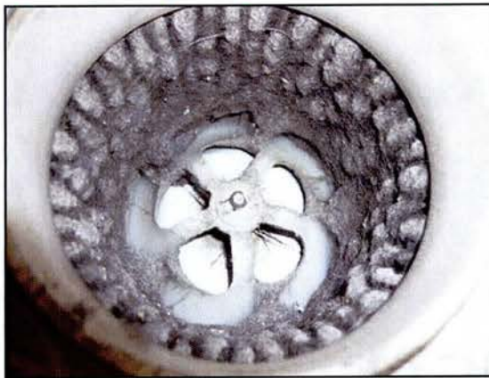
Figure 1. HV Battery Cooling Fan BEFORE Cleaning
