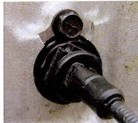
New sensor installed without retaining clip
