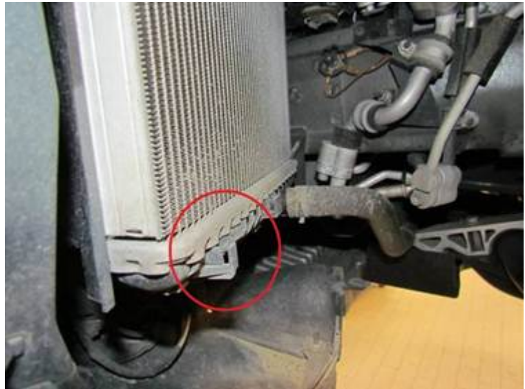
Figure 7. Lower exit air duct attachment point to additional radiator.
