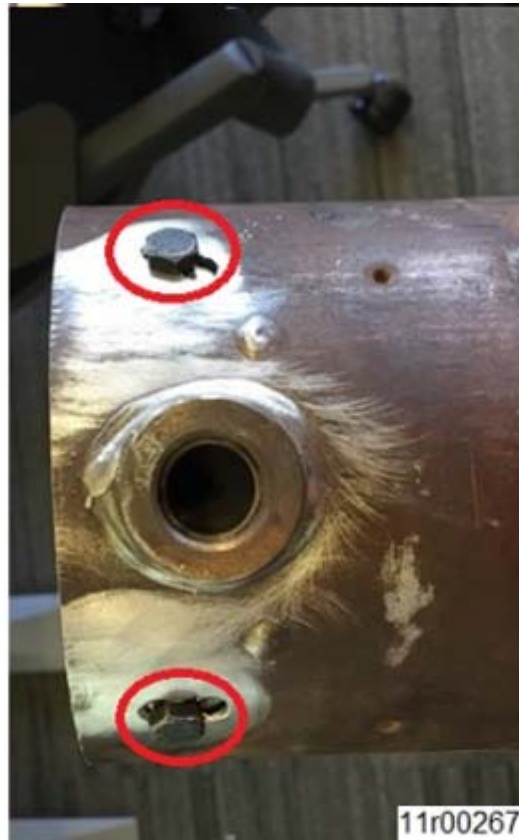
Figure 1, Two Outlet Nox Sensor Bolt-In Water Shield Bolts in the Exhaust Pipe.
