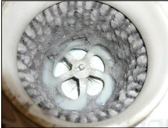
Figure 1. HV Battery Cooling Fan BEFORE Cleaning
